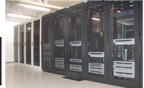
nTOC (network operation center)
