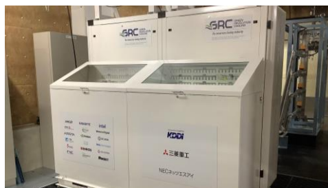
Indoors: Immersion Cooling Unit
