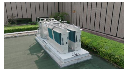
Outdoors: Free Cooling Unit
