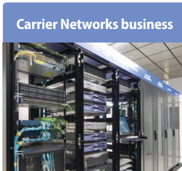
Telecom Carrier Network Equipment
